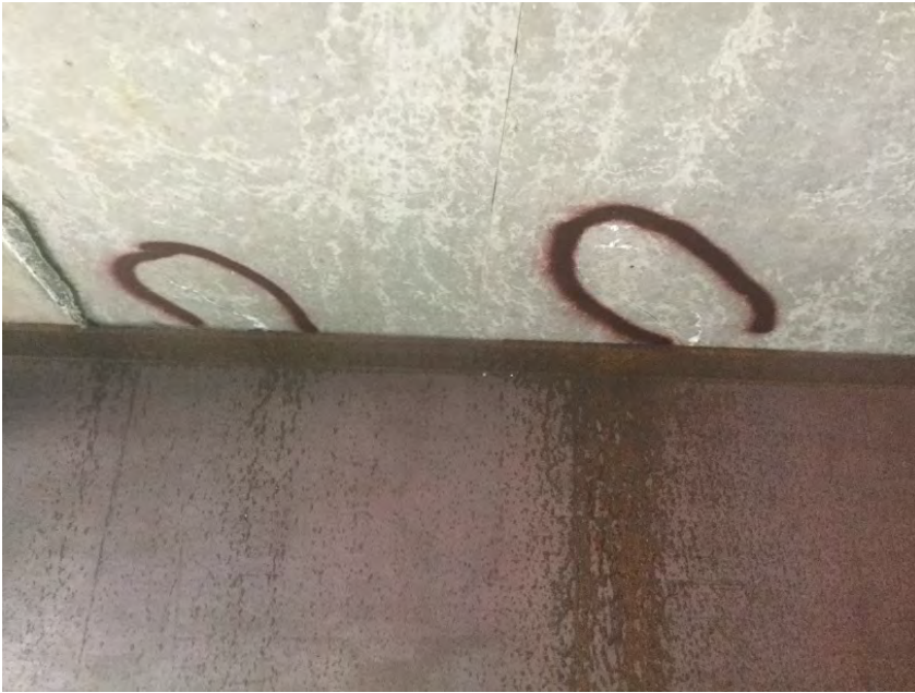
Cracking on underside of girders throughout
