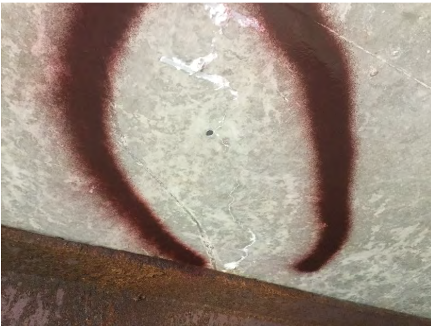
Deck panel cracks
