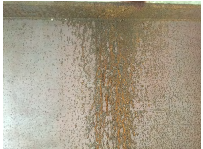
Girders corrosion at deck joint and grout pocket locations
