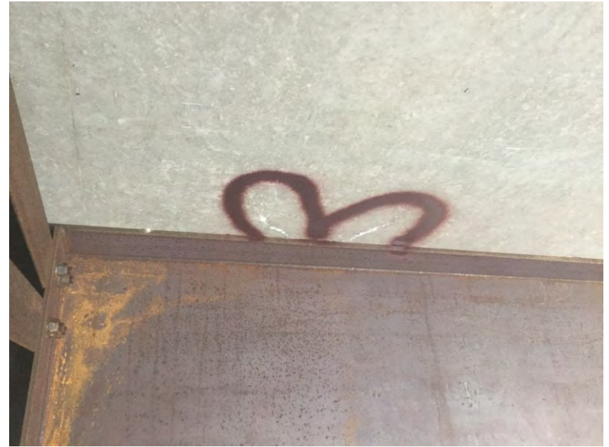
Deck panel cracks
