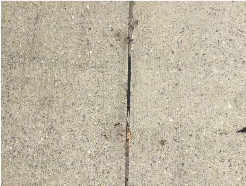
Deck panel joints worn
