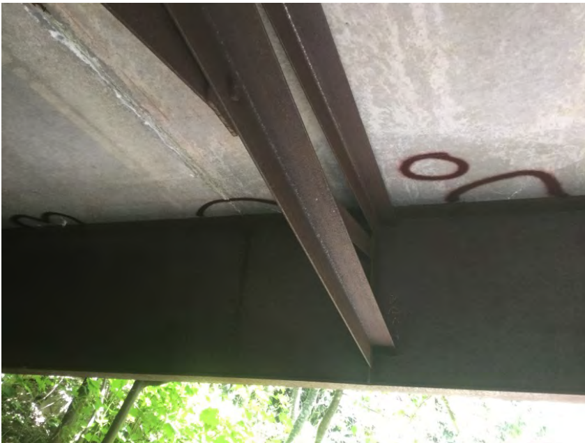
Deck panel cracks
