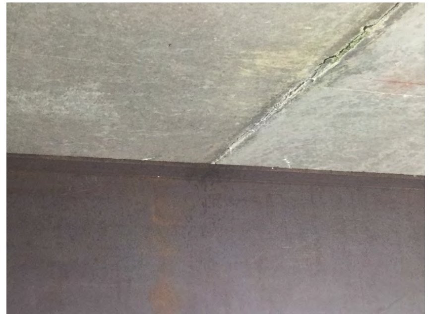
Deck joints cracks
