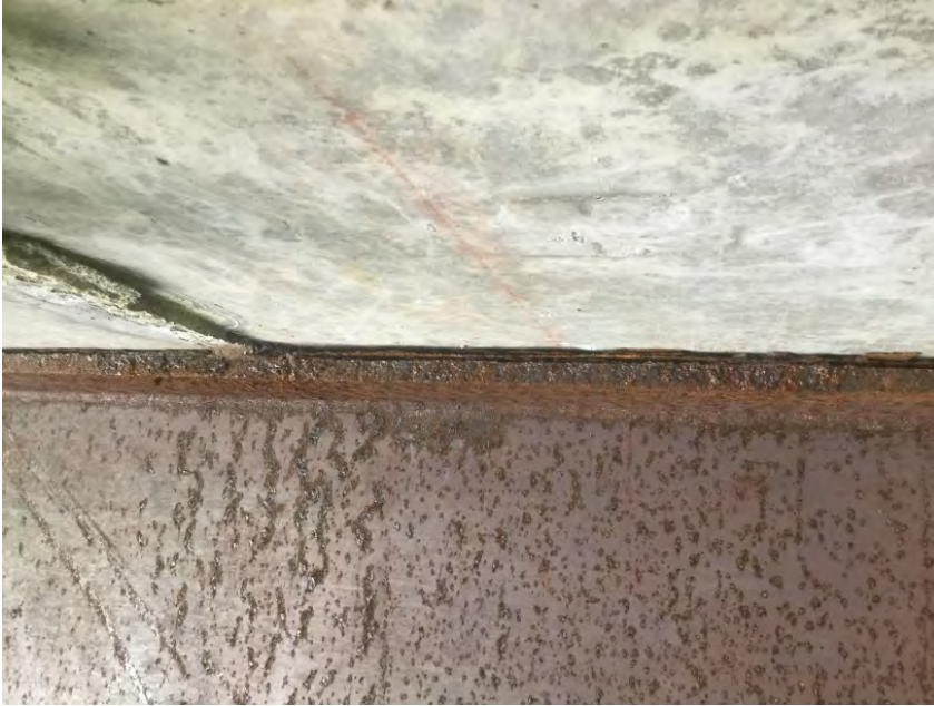
Panels being lifted due to rusting, typical throughout
